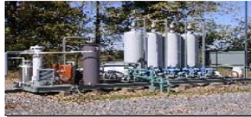
Engelhard Molecular Gate system at a facility in Southern Illinois
