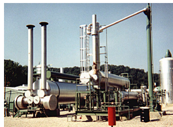
Glycol Dehydrator Unit Source: GasTech
