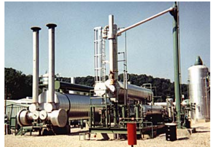
Glycol Dehydrator Unit Source: GasTech
