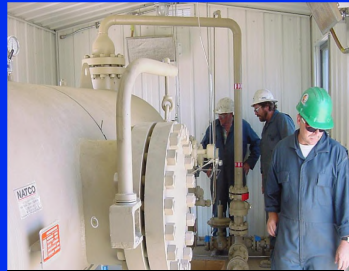
Portable Three Phase Separator, Source: BP
