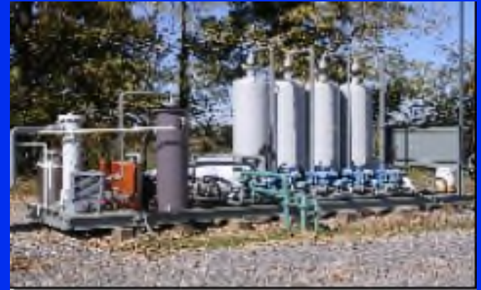
Engelhard Molecular Gate system at a facility in Southern Illinois
