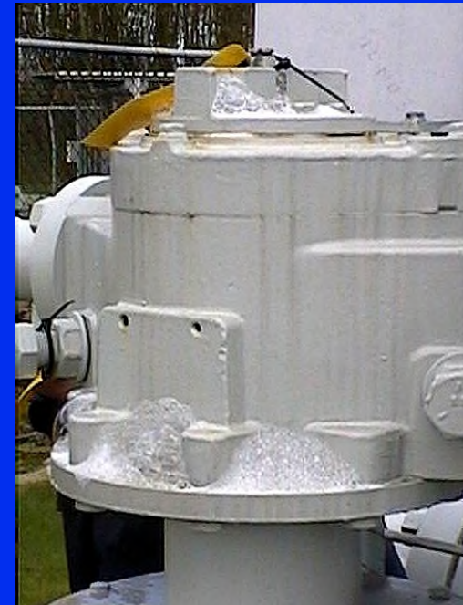
Bubble test on leaking valve
