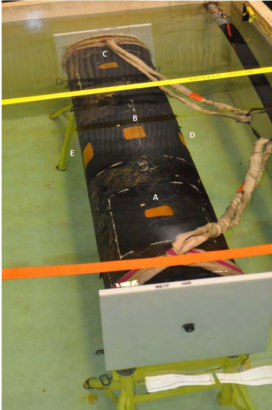
Figure 11: Photograph showing 20" pipe in 40°F water prior to application of epoxy repairs. Repair areas are labeled per Table 1 and Figure 10. Flash rust on exposed areas was removed prior to repair.
