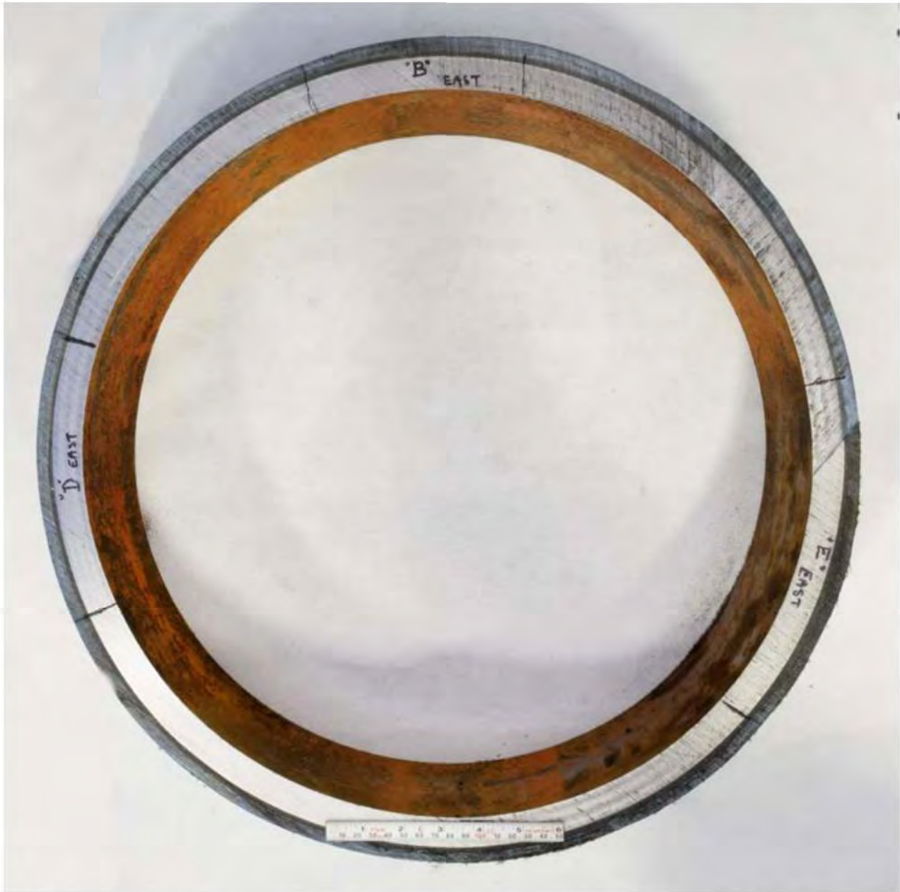
Figure 22: Photograph of cross-sectional ring cut from center of 20" pipe sample containing repair Areas "B/D/E."
