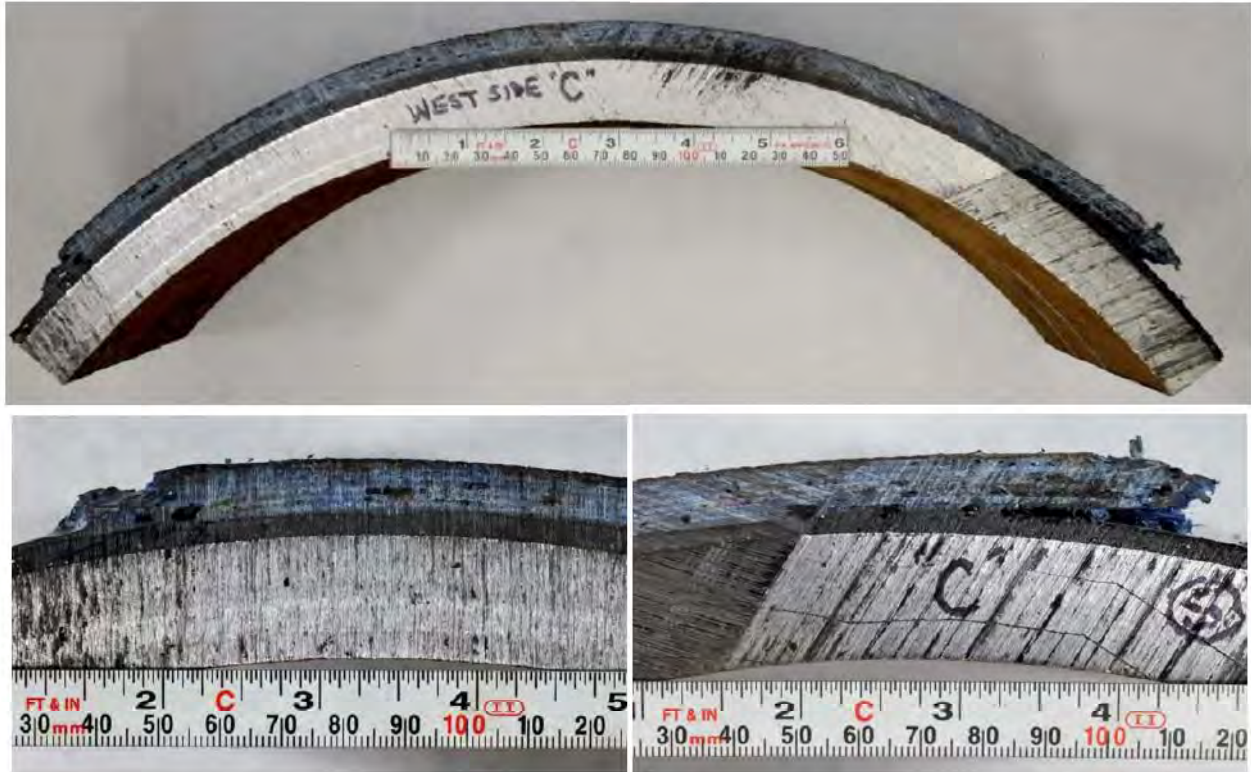
Figure 26: Rough cut cross-section through repair Area “C,” a patch repair where no stricture banding was used. While center of repair was well adhered to pipe wall, perimeter of patch was disbonded from pipe.
