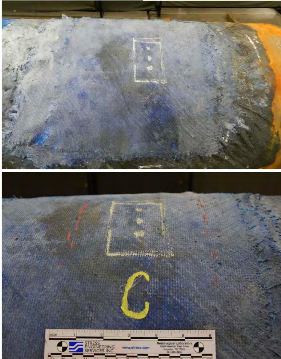
Figure 19: Photographs showing patch repair at Area “C” where no stricture was applied.
