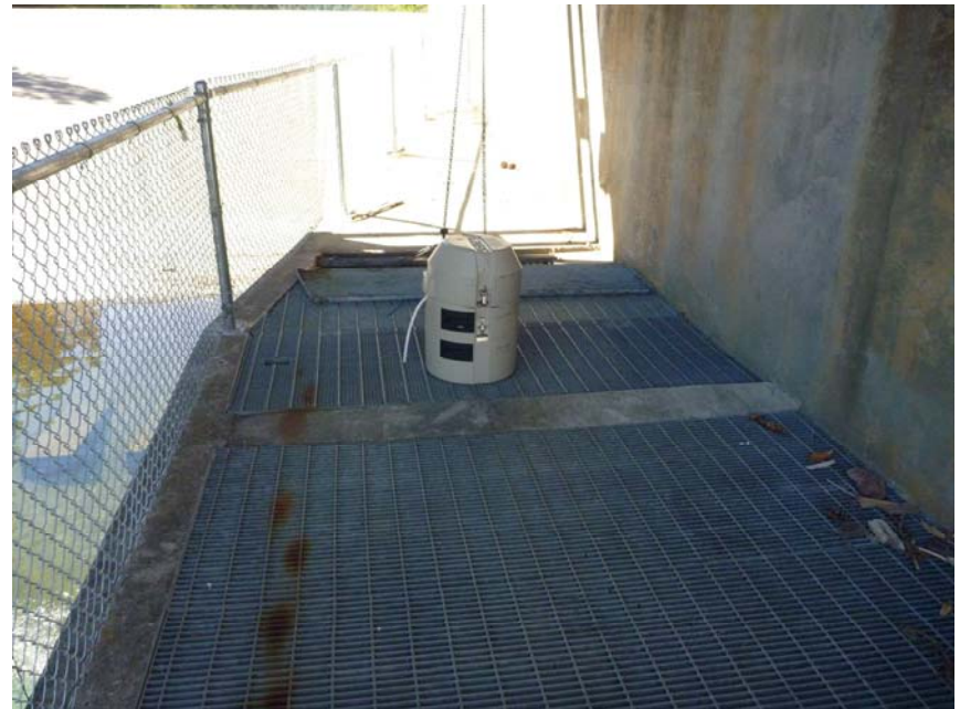
22- Automatic sampler deployed at LNFH effluent location
