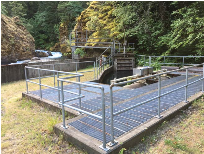
1 – LWSNFH Influent water location
