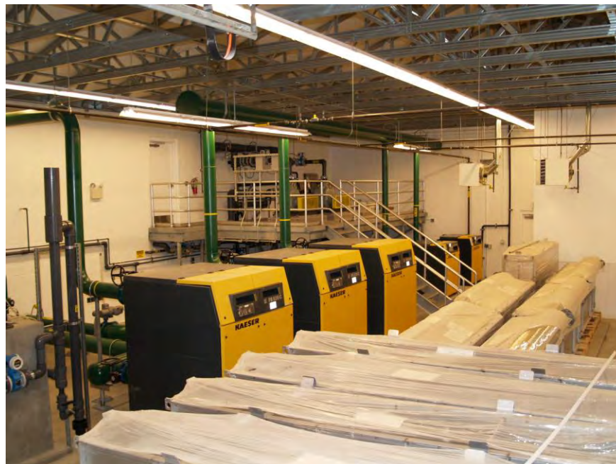
Figure B-5: Photograph of aeration blowers at the Avimor Water Reclamation Facility.
