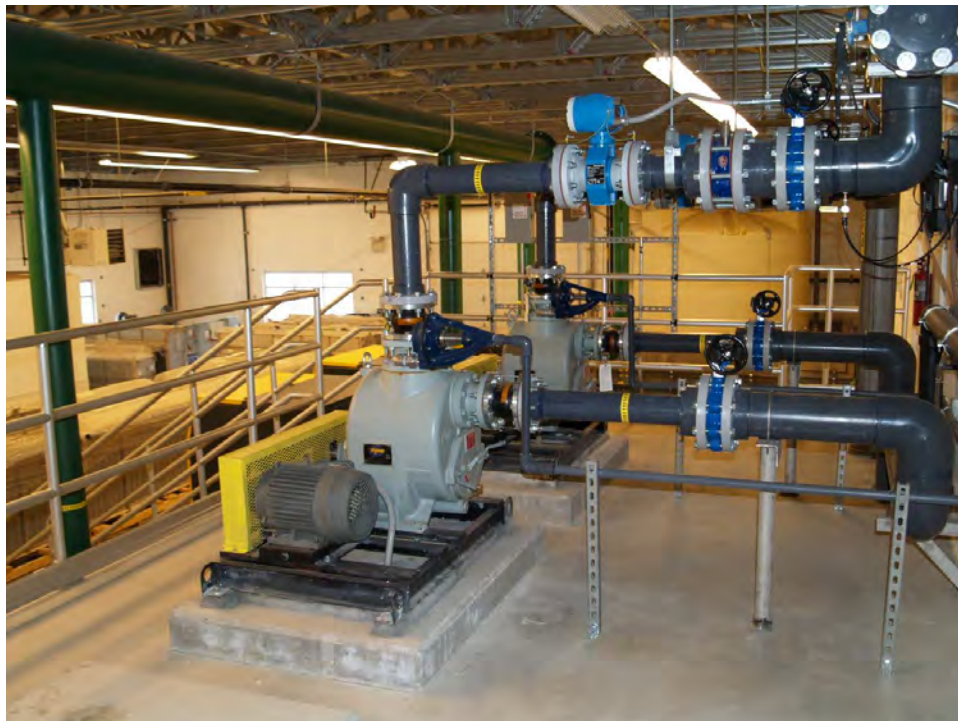
Figure B-7: Photograph of permeate pumps at the Avimor Water Reclamation Facility.
