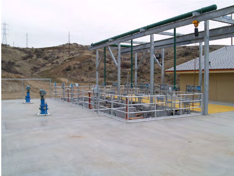
Figure B-6: Photograph of anoxic, aeration, and MBR chambers at the Avimor Water Reclamation Facility.
