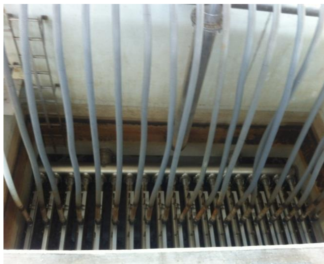
Figure 6-2. Submerged MF membranes at OCGWR
