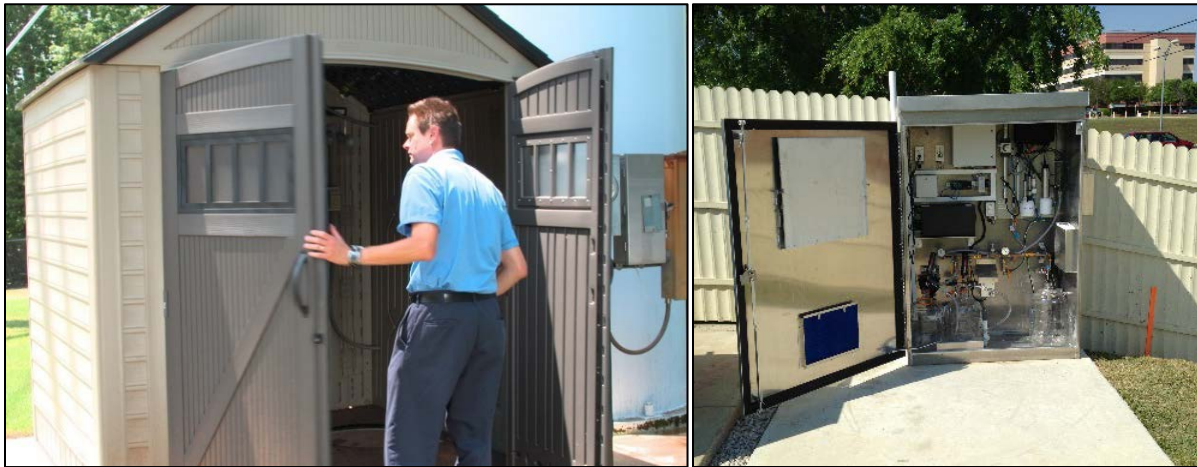
Figure 2-4. Enclosed Station Installations (Prefabricated and NEMA Enclosures)
