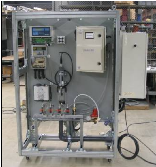
Figure 2-3. Free-Standing Rack Installation
