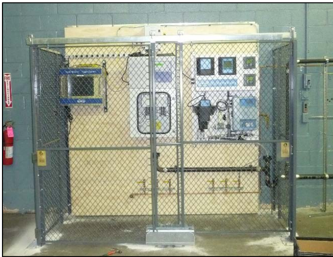
Figure 2-2. Wall-Mounted Rack with Protective Cage
