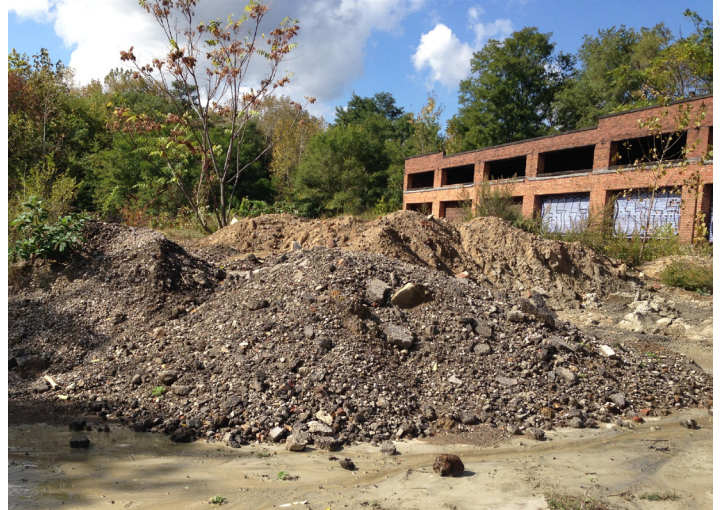
Construction/demolition debris waste piles observed along the corridor.
