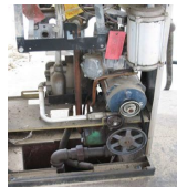
Suction piping system
