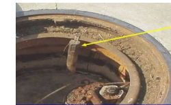
Tank top sump sensor installed too high
