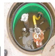
Tank top sump full of liquid
