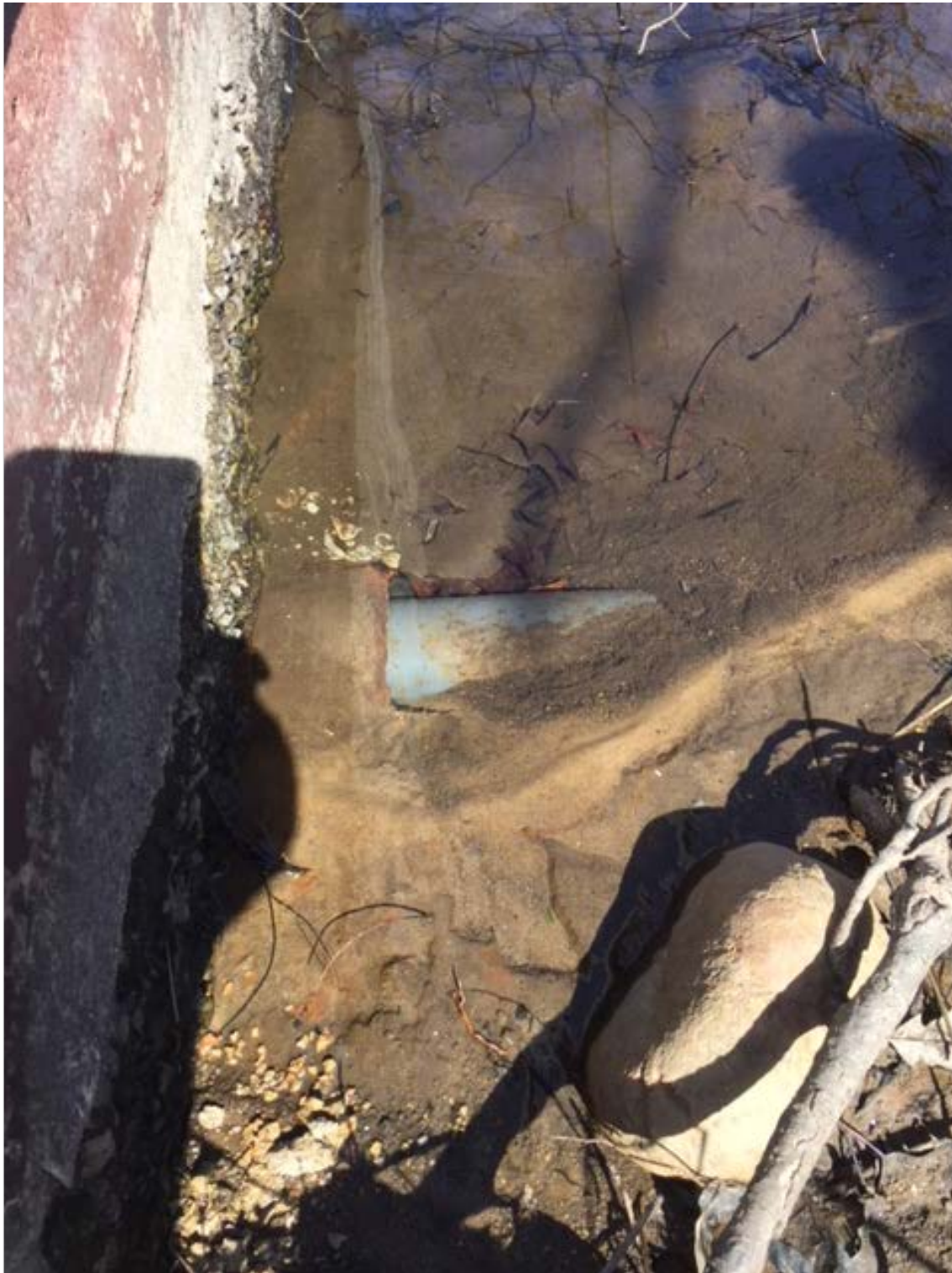
Figure 9: Water Entering Screen Well of Intake Structure
