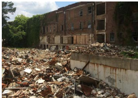
Debris pile in the basement area of the Old Davis Hospital demolition site as of June 2016. (EPA photo)
