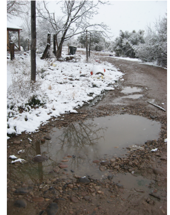
The CWISA Program addresses wastewater deficiencies such as this failed septic system.
