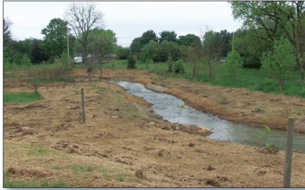
Figure 2. The new stream channel diverts water around a small concrete dam, now buried.
