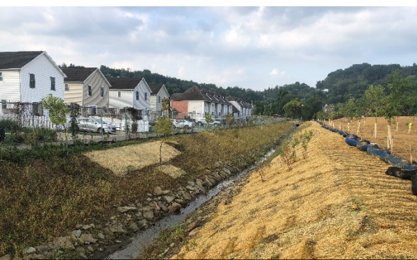
Old Bull Run Tunnel was removed to daylight the stream on the eastern boundary of the Former Jeannette Glass site.
