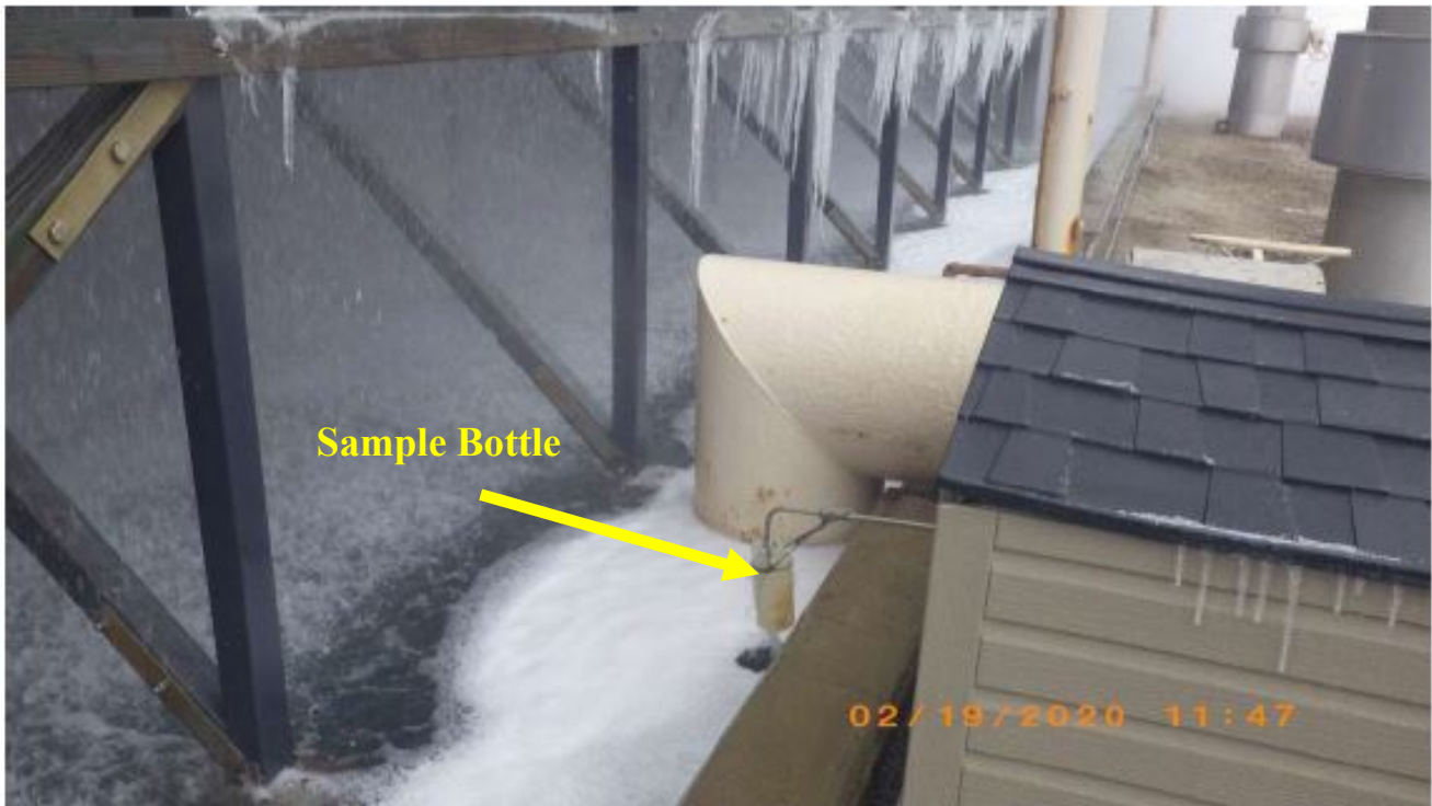
Figure 7 - Cooling Tower Basin Blowdown-Monitoring Station
