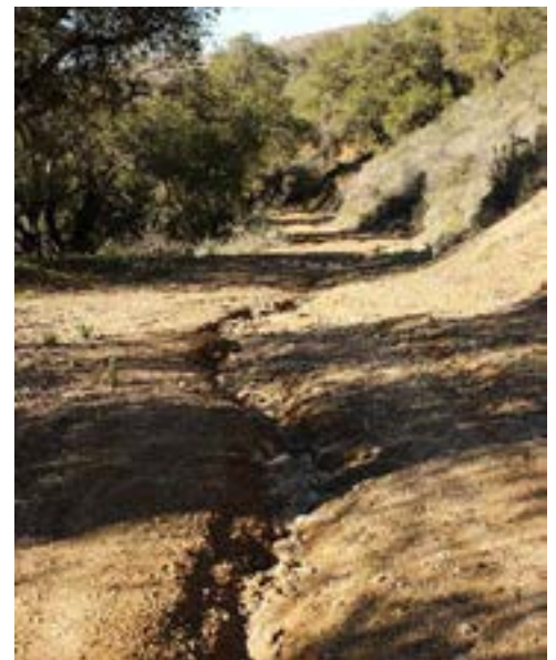
The La Jolla Band of Luiseño Indians is using EPA funding to stabilize Cedar Creek Road. The road is a high priority for management measures because erosion is likely contributing sediment, metals, and hydrocarbons to the San Luis Rey Watershed.
