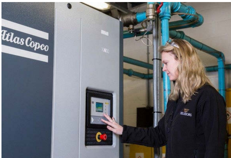
Compressor Pressure Reduction
