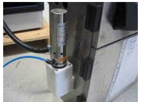
Compressed Air Cabinet Cooler
