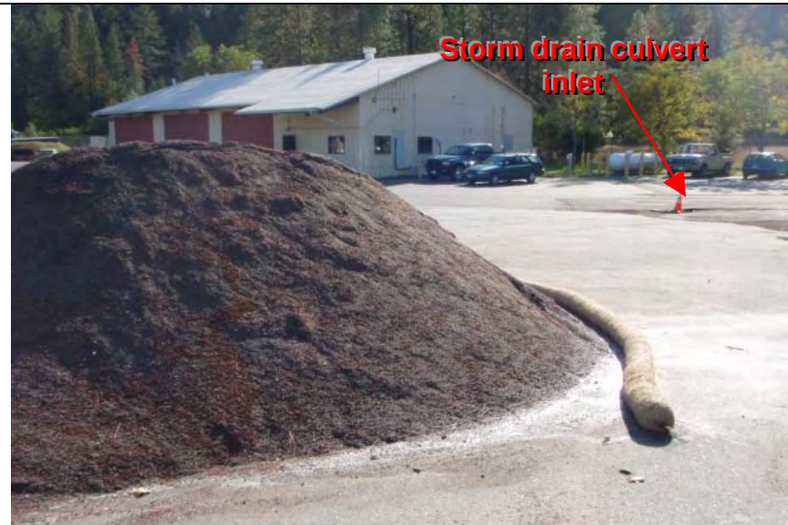
Photograph 6 – Inappropriate application of straw wattle BMP
