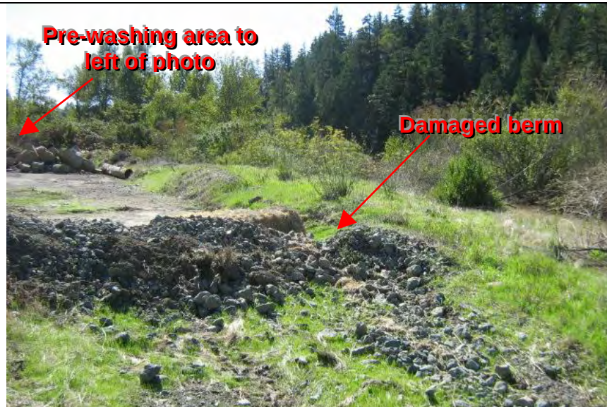
Photograph 7— Damaged berm shown in Photograph 6
