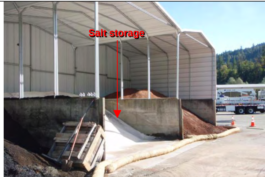
Photograph 8 – Inappropriate application of straw wattle BMP
