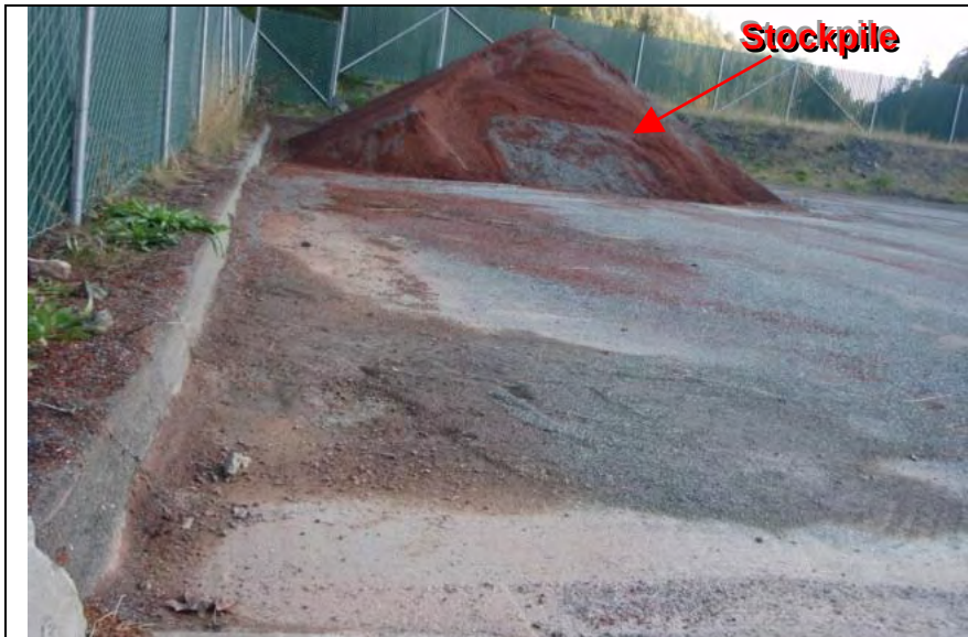
Photograph 1 – Stockpile without BMPs for coverage or containment
