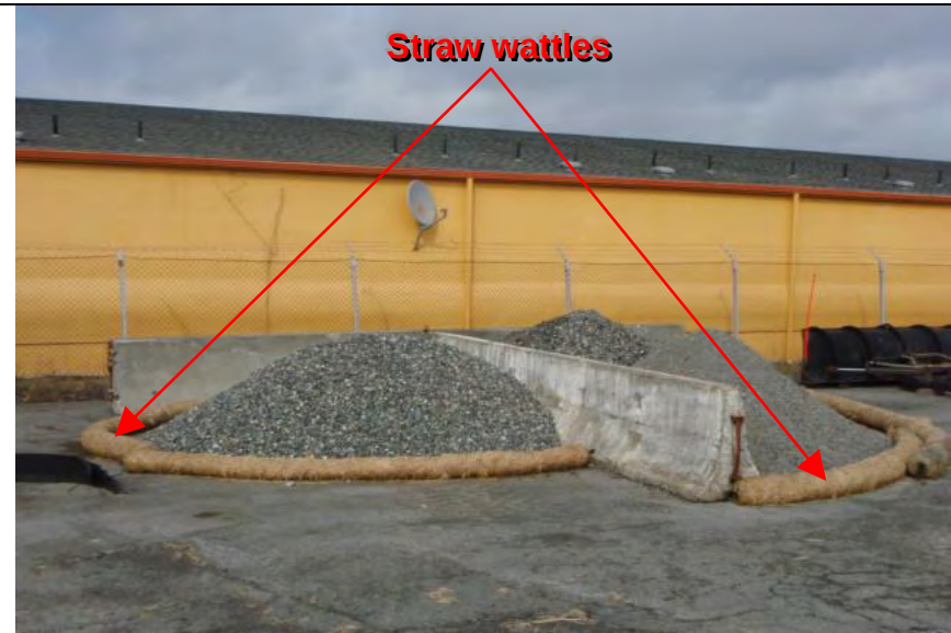
Photograph 10 – Inappropriate application of wattles on impervious surface
