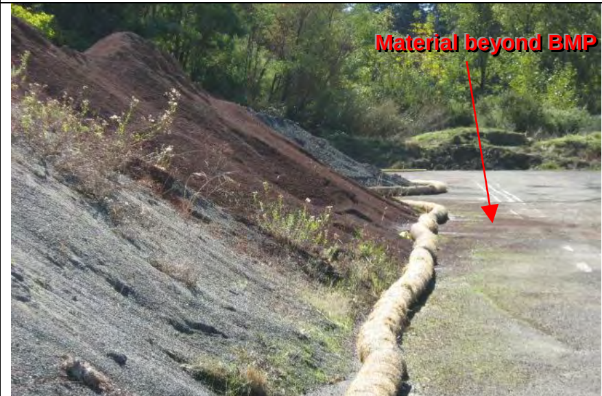
Photograph 8 – Inappropriate application of wattles on impervious surface
