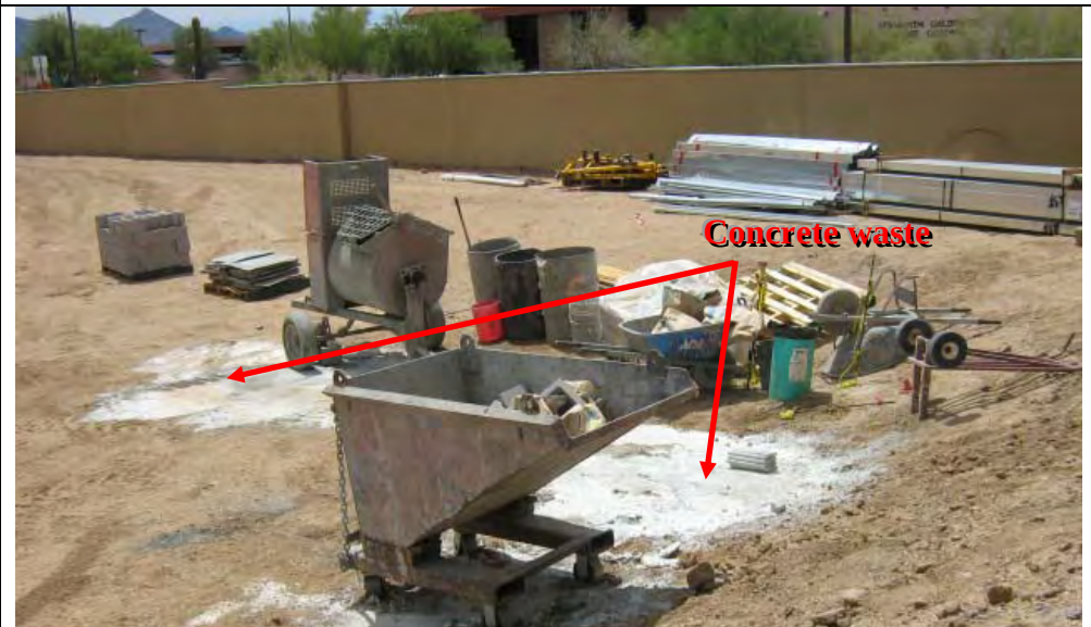
Photograph 4 – Potential source of the illicit discharge
