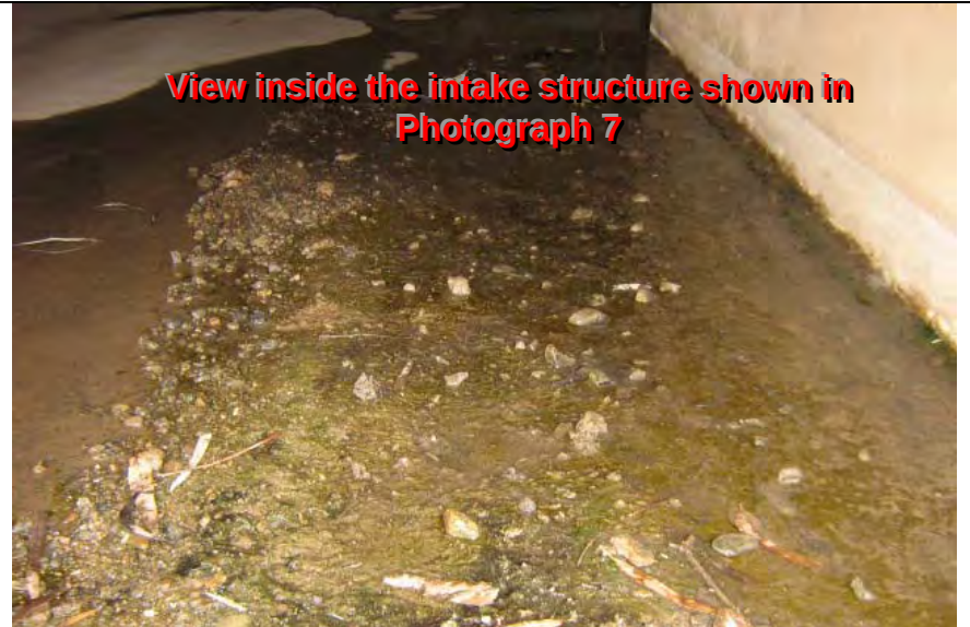
Photograph 8 – Sediment and debris accumulation in intake structure
