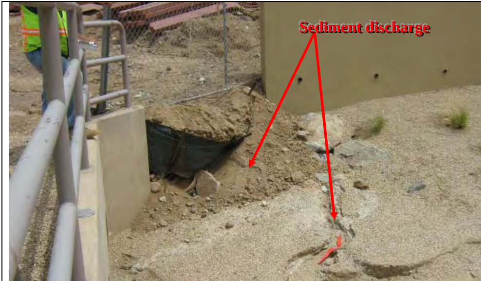
Photograph 9 – Silt fence failure and offsite sediment
