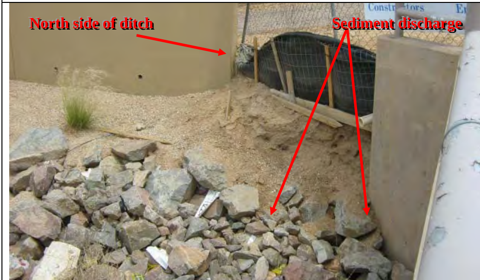
Photograph 7 – Silt fence failure and offsite sediment
