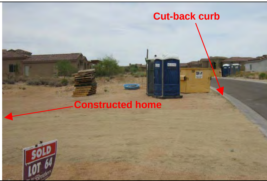
Photograph 3—Lack of perimeter control BMP
