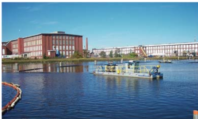
Dredge in upper New Bedford Harbor (Oct. 6, 2004). Aerovox was located in the building in the back (center to right). Photo courtesy of EPA Region 1
