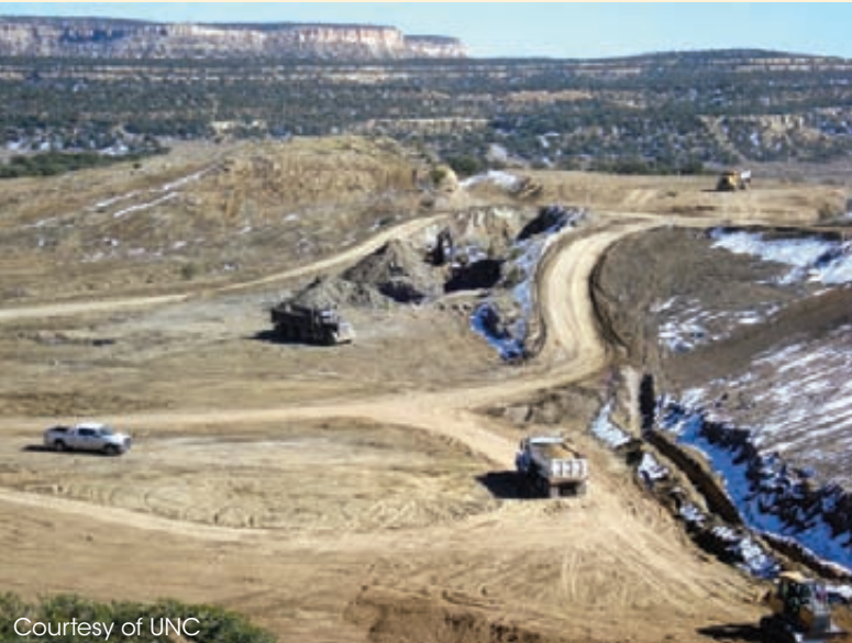
Courtesy of UNC Cleanup at Northeast Church Rock mine
