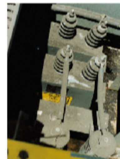
PCB Capacitors in a mine power center
