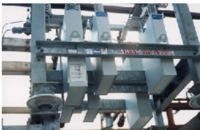
PCB marked capacitor
