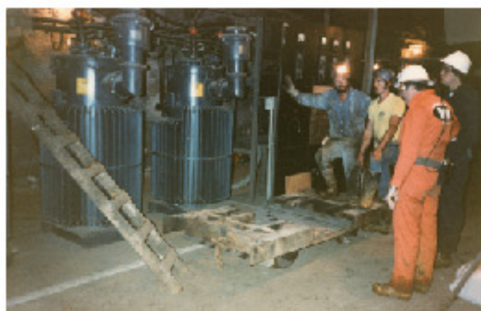
76 gallon PCB transformers (cylindrical objects with cooling fins) with PCB marks in an underground mine
