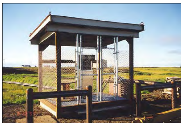
Figure 3-2. Fencing around a dispenser pump.
