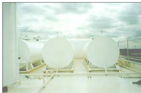
Figure 7-3. Shop-built containers elevated on saddles.
